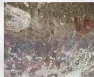
Damage: Panel used for target practice
