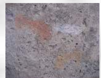
Damage: The art has been scratched away
